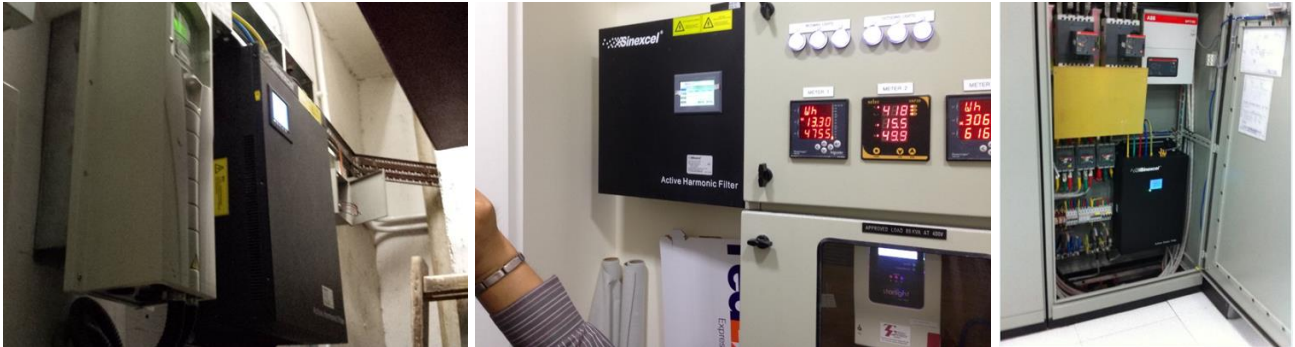
Fig 1. The compact size wall mount type of AHF being installed in confined space in electrical riser or tenant meter closet
